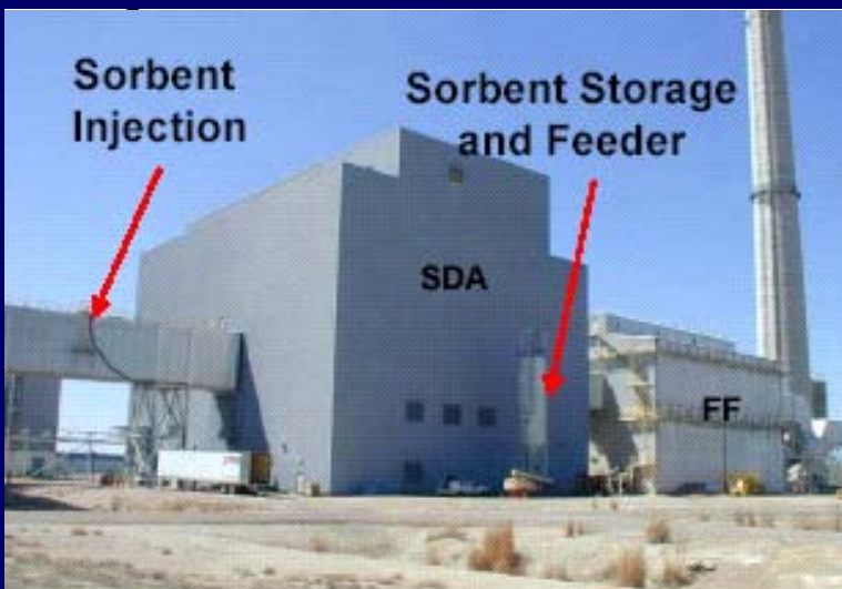
Power plant with SDA and Activated Carbon Injection upstream of an existing fabric filter.
