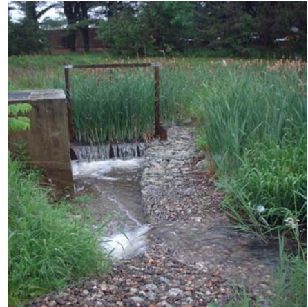
Stormwater Wetlands Outlet Structure during a storm (May 2003)
