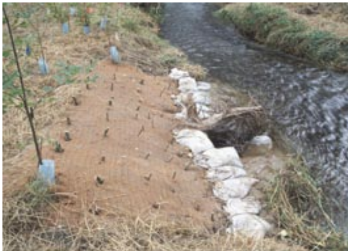
Streambank stabilization project along Dogfish Creek, Washington, showing root wads and plantings. Source: NRCS
