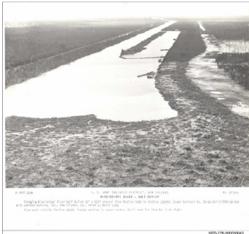
9 July 1958 Photograph: Looking due east towards Paris Road in the background. Note cypress tree removal before dredging. Based on the three story height of dredger, trees were about 40 feet tall. The figure also shows extensive cypress forest in the Central Wetlands. (Day and Shaffer, 2009)
