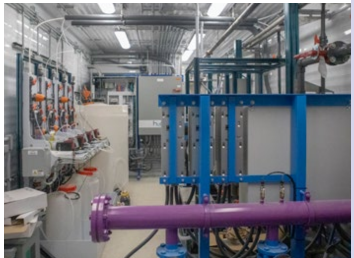
▲ Austin's Closed-Loop Advanced Reclaimed Assembly (CLARA) system can treat up to 5,000 gallons of wastewater per day from the building's sinks, toilets and drinking fountains. CLARA is a hybrid membrane system with six stages of biological, physical, and chemical treatment. Photo courtesy of Austin Water.
