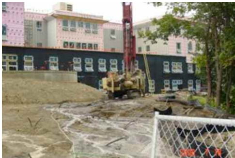
The University of Maine at Farmington’s Education Center during construction shows the borehole drill rig and the paired ends of some geothermal loops protruding from the ground.
