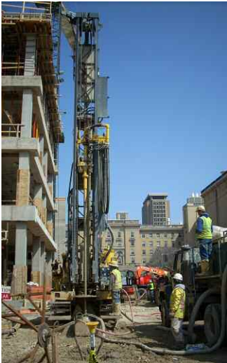
Drill rig at the University of Wisconsin-Madison drilling through 300 feet of soil and bedrock to make one of 75 boreholes for a closed loop GHP system.
