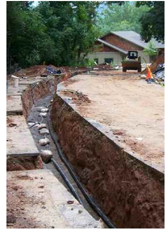
Outside Warren Wilson’s Jensen building, plastic piping that interconnects the loop field is laid out in a trench and then buried below the frost line.
