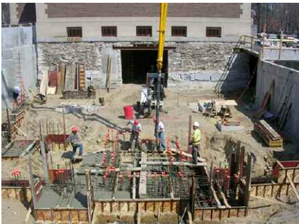
The new underground space outside Bowdoin College's Walker Art Building now houses the visitor services department.
