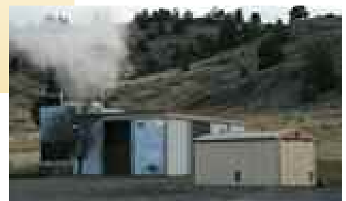
Steam rises from the new 280 kW geothermal power plant at the Oregon Institute of Technology.
