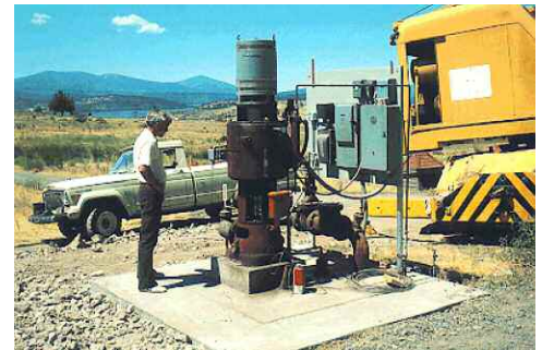
One of three wells that provides 192° F groundwater for the OIT system.
