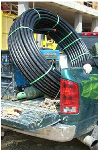
Coil of 600 feet of plastic tubing needed for one 300-foot deep loop in a GHP system. Inset shows the U-shaped end that goes to bottom of the borehole.
