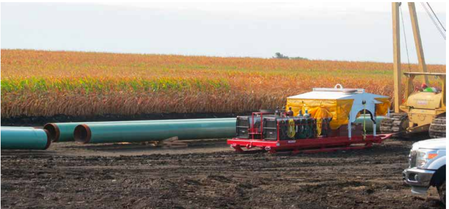
CONSTRUCTION OF FLANAGAN SOUTH PIPELINE IN LIVINGSTON COUNTY, ILLINOIS. PHOTO CREDIT: JENNA DOOLEY/NORTHERN PUBLIC RADIO
