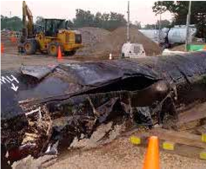
PIPELINE RUPTURE IN ENBRIDGE'S LINE 6B. PHOTO CREDIT: NATIONAL TRANSPORTATION SAFETY BOARD.
