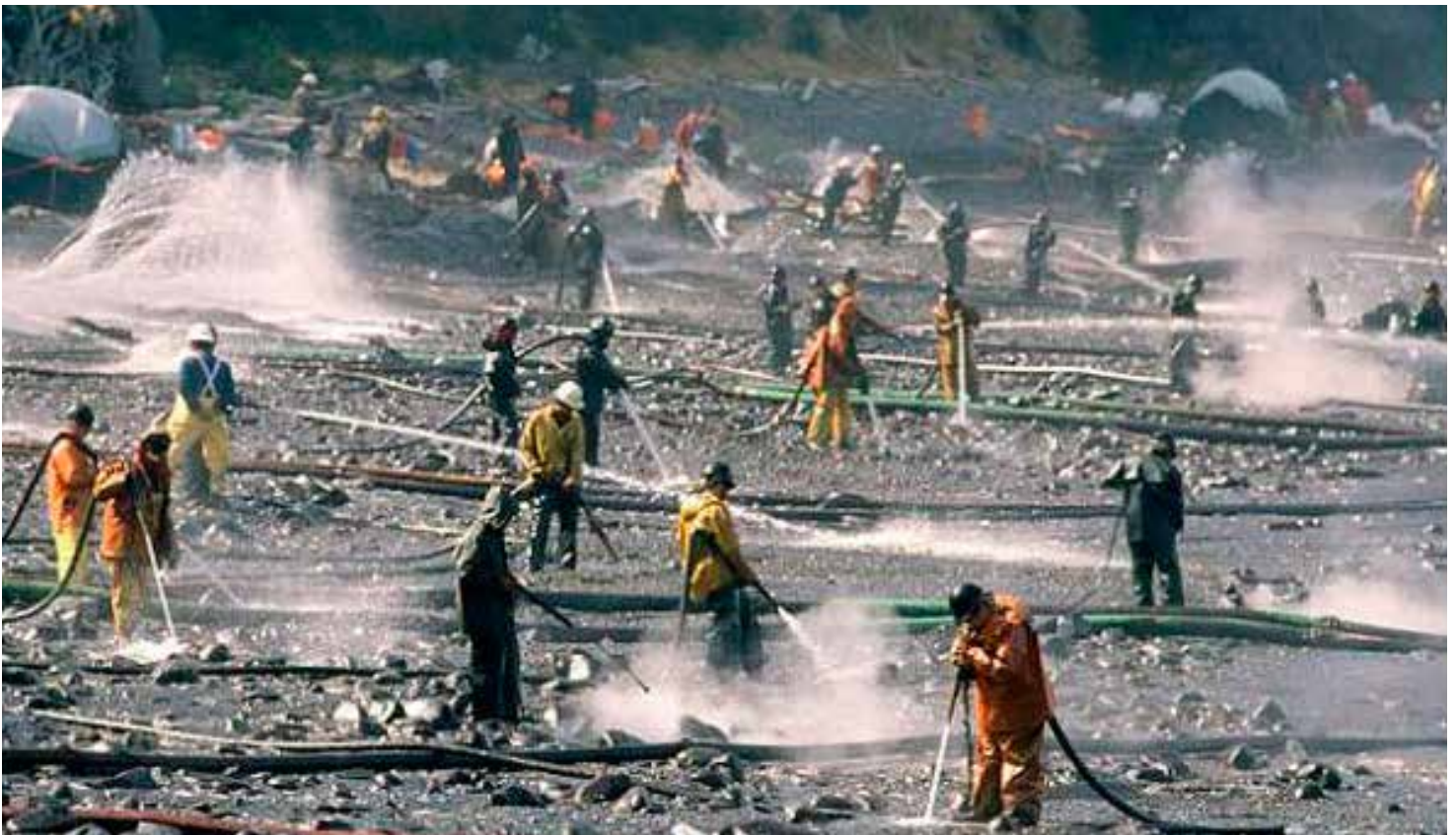
TAR SANDS SPILL CLEAN-UP CREWS AFTER 2010 KALAMAZOO RIVER SPILL. PHOTO CREDIT: JACK MCNEARY
