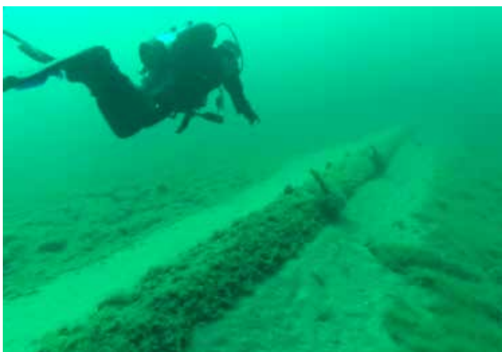
A DIVER POINTS OUT RUSTED METAL STRAPS ON LINE 5 BENEATH THE STRAITS OF MACKINAC. PHOTO CREDIT: STILL FROM VIDEO PRODUCED BY THE NATIONAL WILDLIFE FEDERATION.
